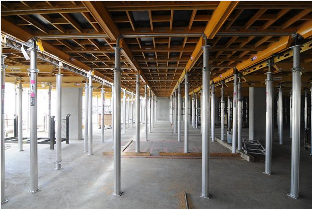
Andersen Construction is preparing to pour the deck for the building's parking garage, which will accommodate 249 vehicles.
