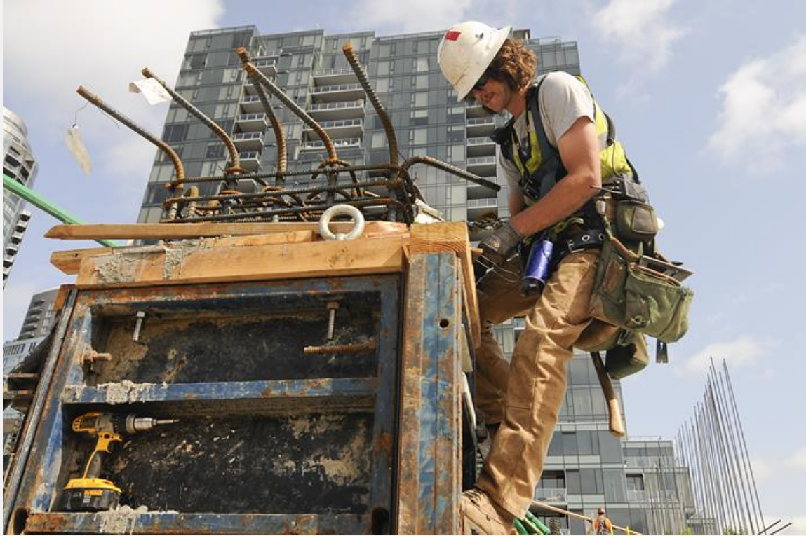
Bjorn Drake, a carpenter with Local 503, installs formwork around a rebar column.
